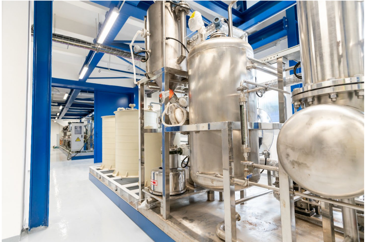
Crystallization Module of the Chvaletice Manganese Project Demonstration Plant
