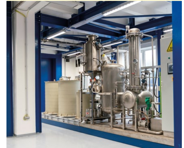
Image: HPMSM crystallization module at the newly installed Demonstration Plant.
